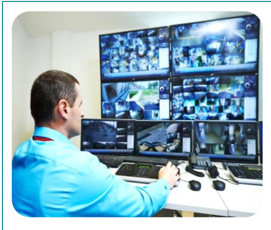
Figure 63: CCTV Control Room
